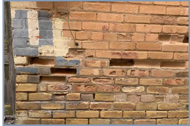
Inappropriate replacement materials can damage surrounding materials.
