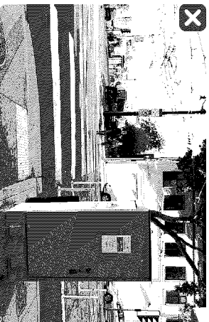
Utilities located along the ground floor and at street corners impede the line of sight for both motorists and pedestrians.
