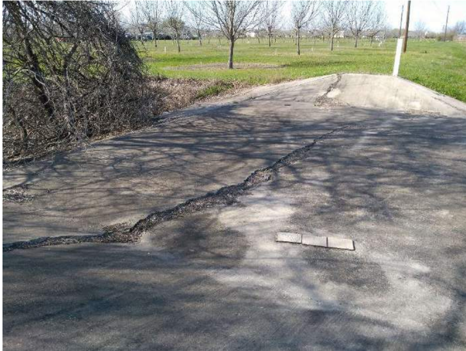
OVERFLOW STRUCTURE (NOTE CONCRETE CRACKING AT OVERFLOW WEIR)
