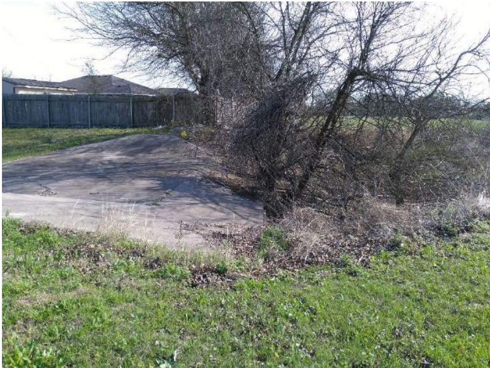
OVERFLOW STRUCTURE (NOTE OVERGROWN AT DOWNSTREAM)
