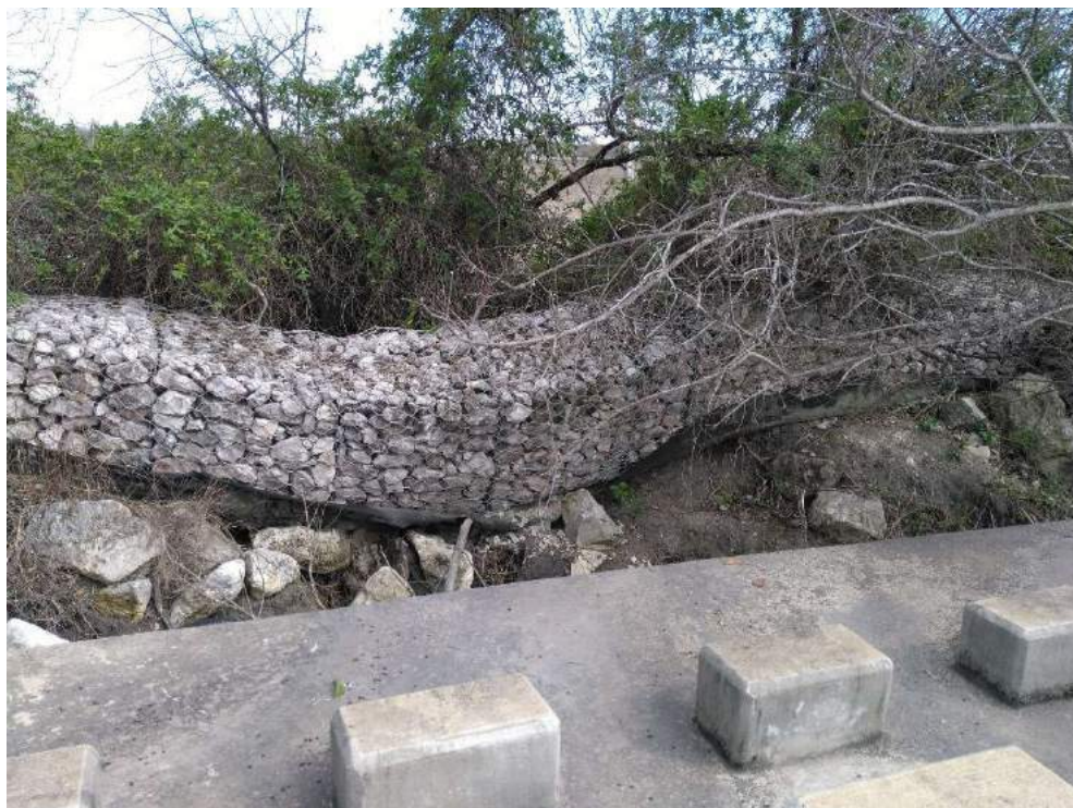
OUTFALL STRUCTURE UNDERMINING
