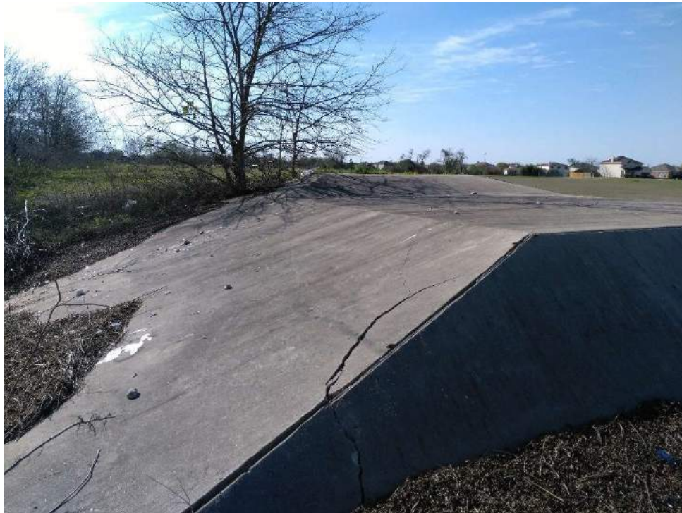
OVERFLOW STRUCTURE (CONCRETE CRACKING AND SEPARATION)
