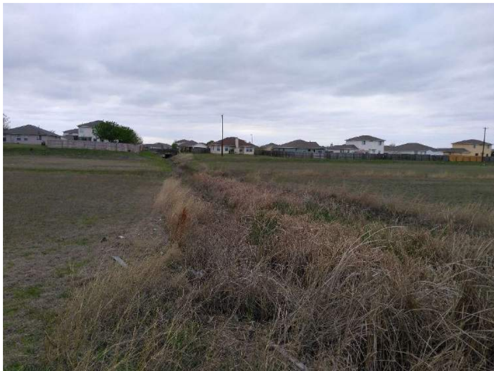
TRICKLE CHANNEL OVERGROWN WITH VEGETATION
