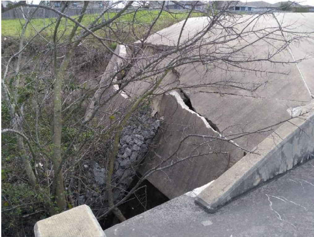
OUTFALL STRUCTURE UNDERMINING
