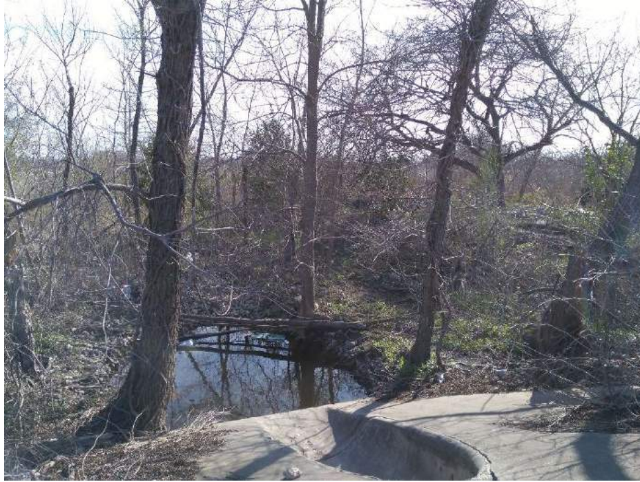
OVERFLOW STRUCTURE (STANDING WATER, UNDERMINING AND OVERGROWN VEGETATION AT DOWNSTREAM)
