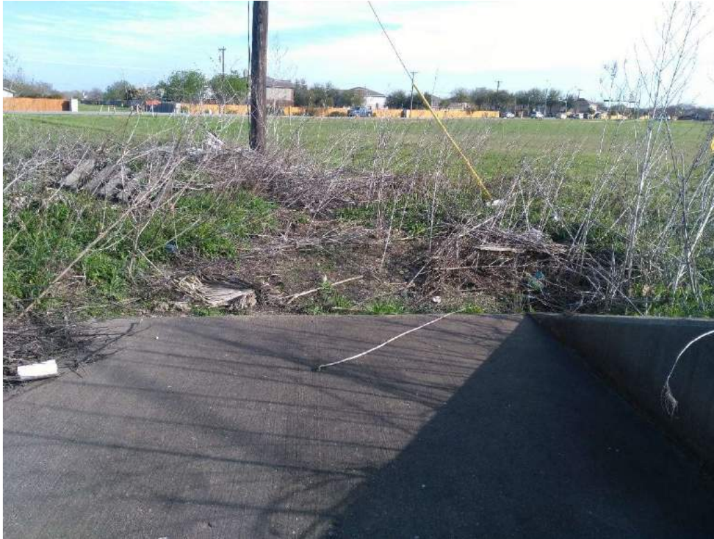
OVERFLOW STRUCTURES (NOTE SLIGHT UNDERMINING AT DOWNSTREAM)
