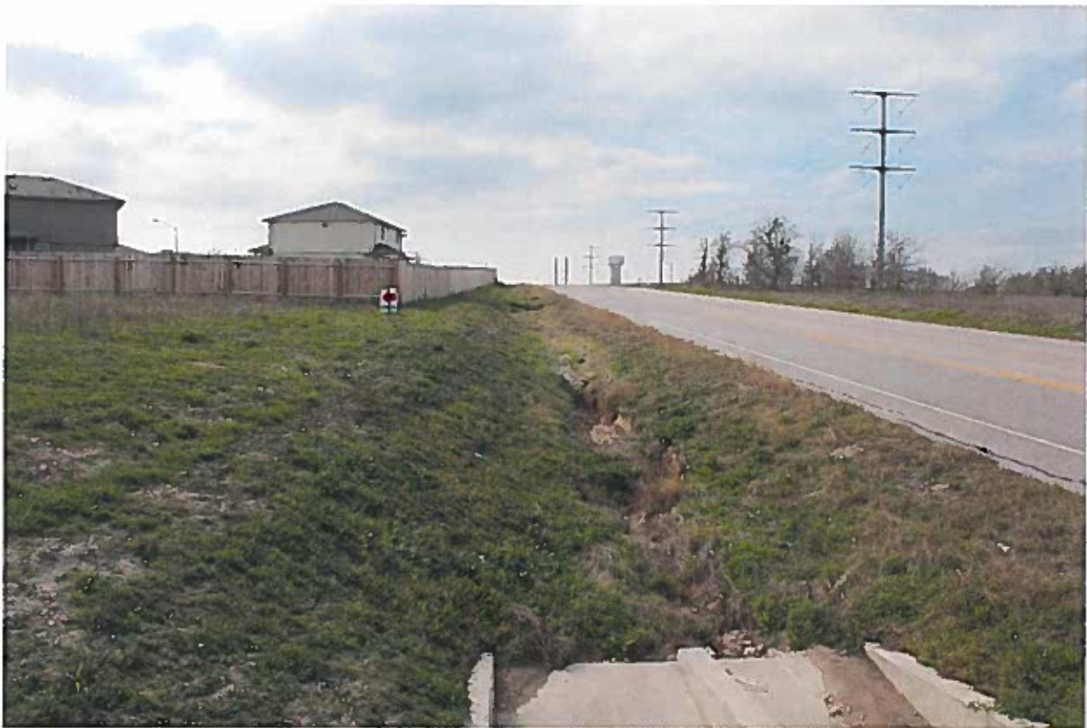
Photo 2 – Looking west on southside of Limmer Loop towards Cottonwood Creek Elementary (please note there are no school zone signs on Limmer Loop)
