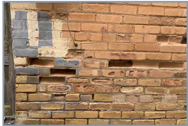
Inappropriate replacement materials can damage surrounding materials.
