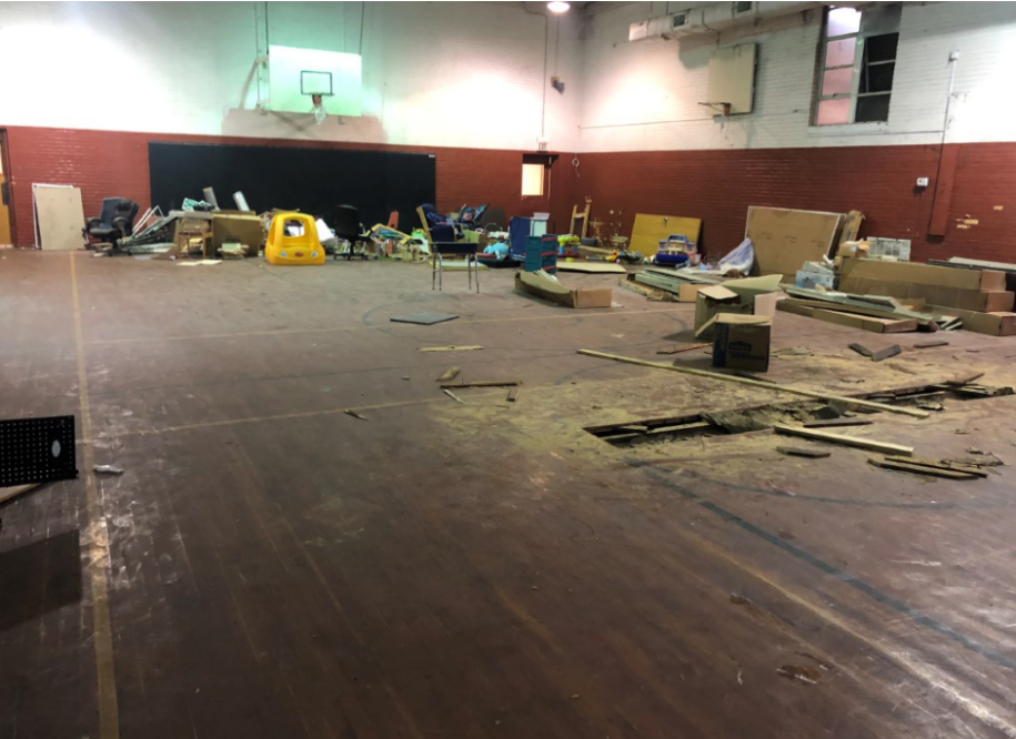
ITEM NO. 2: WOOD FLOORING. SALVAGED MATERIAL WILL BE TAKEN FROM MIDDLE AS EDGES HAVE WATER DAMAGE
