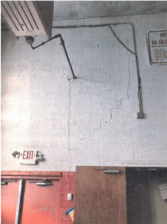
Photo 16 - CMU crack in west wall.
