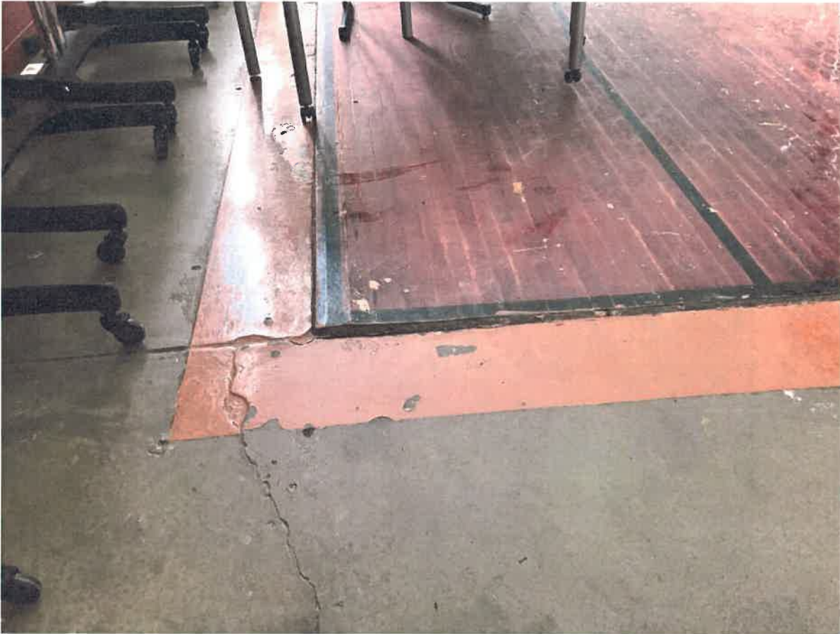
Photo 21 - Southeast corner of basketball court floor.
